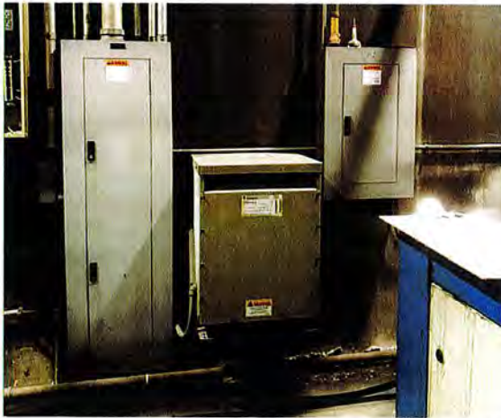
Panel PP1 (480V), 15Kva Transformer and Panel CP-1 (208V)
