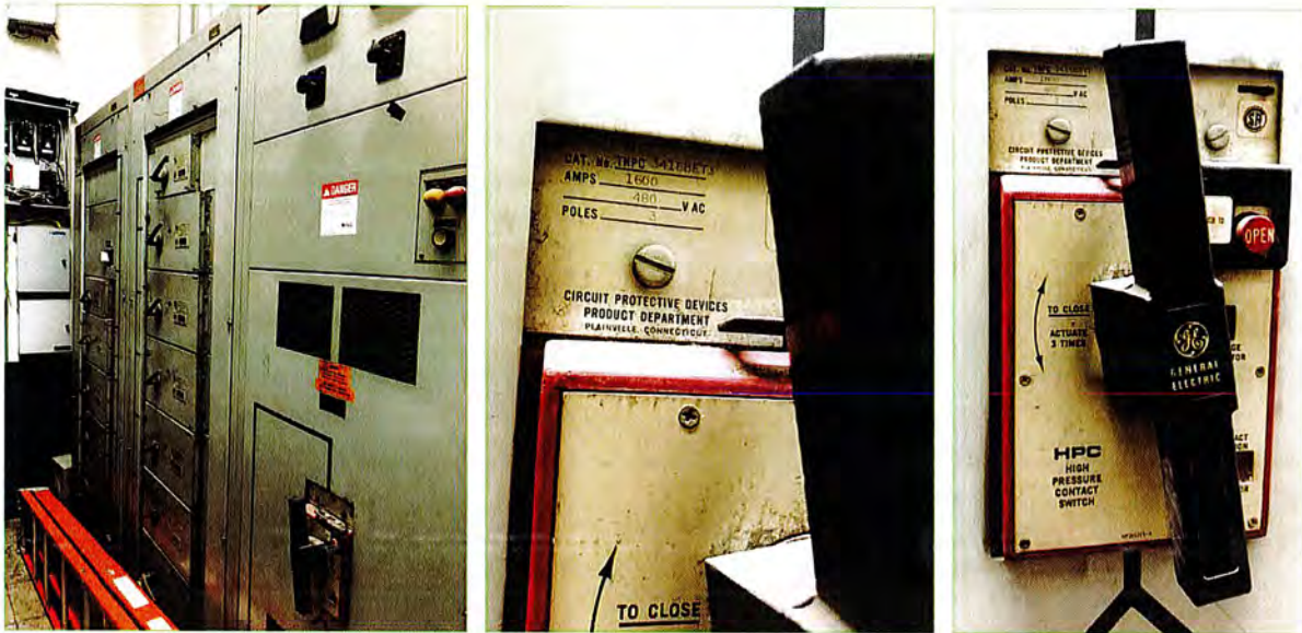
Main Switchboard SW2 1600 amp Rated, 1200 amp Fused
