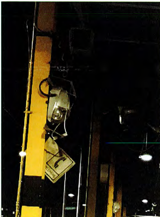
Wire Guard (appears damaged)
