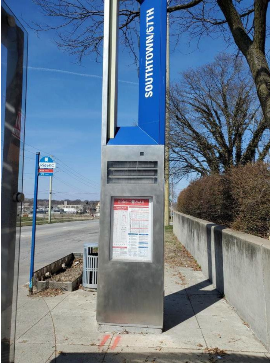
67 TH AND TROOST NORTHBOUND STATION MAX KIOSK EXISTING MAX KIOSK DOES NOT APPEAR TO BE ACTIVE NOTE EXISTING POWER MARKINGS ON GROUND
