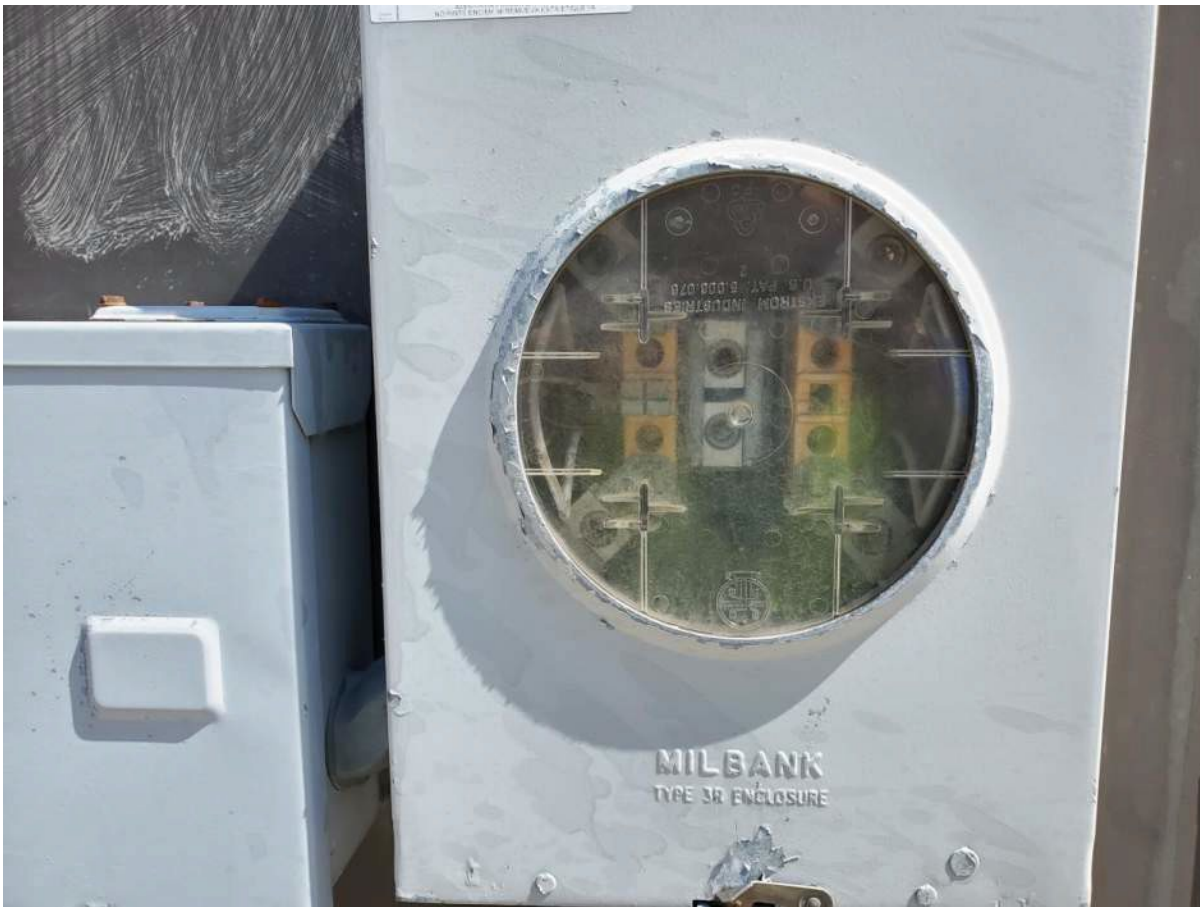
EXISTING ELECTRIC METER AT 9 TH AND OAK NORTHBOUND
